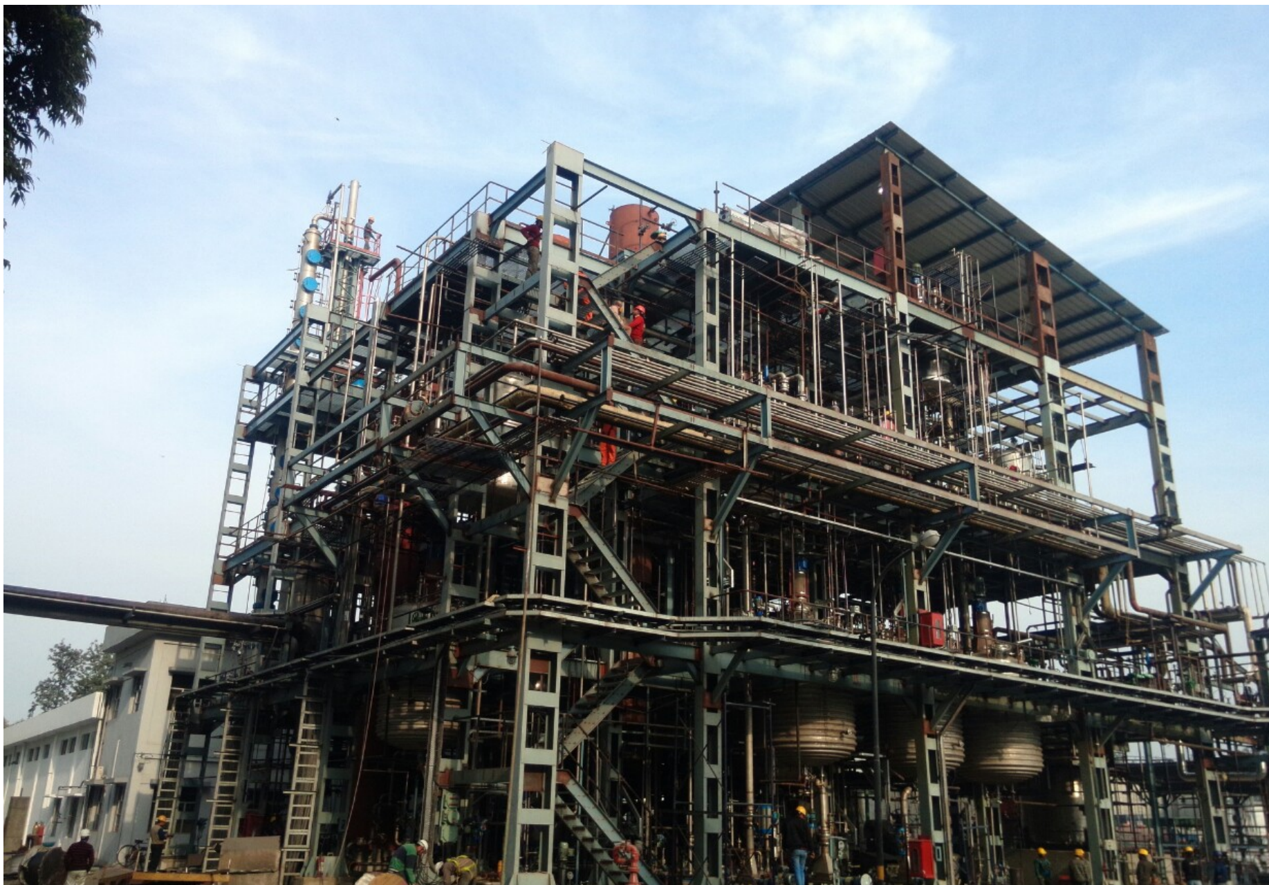
Pilot plant for production of ethanol from lignocellulosic waste, Kashipur, India. Designed by ICT Mumbai Centre for Energy Biosciences. Photo: courtesy of Prof A June 2018
